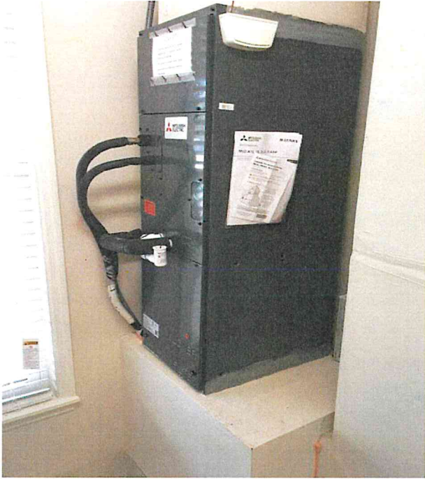
Figure 029: HVAC unit at amenity center.
